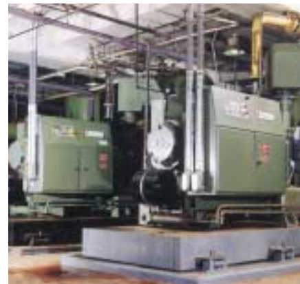
Two 300 HP (225 KW) Turbo Air® Compressors installed a water treatment facility.
