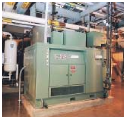
One 300 HP (225 KW) Turbo Air® Compressor installed at a major university for instrument air.
