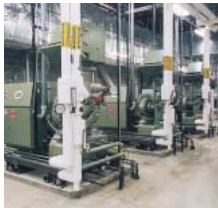
Three 200 HP (150 KW) Turbo Air® Compressors installed at an electronics facility. Three 500 HP (370 KW) Turbo Air® Compressors are also installed.
