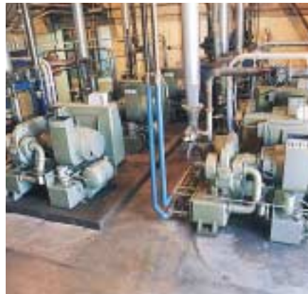
Six 350 HP (260 KW) Turbo Air® Compressors installed at an automotive facility.
