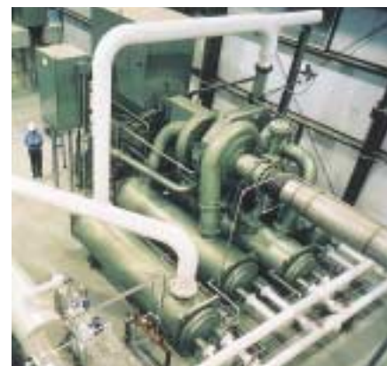
One 10,000 HP (7455 KW) MSG® Air Compressor installed at an air separation facility. One 11,000 HP (8200 KW) MSG® combination Nitrogen Feed/Recycle Compressor is also installed.
